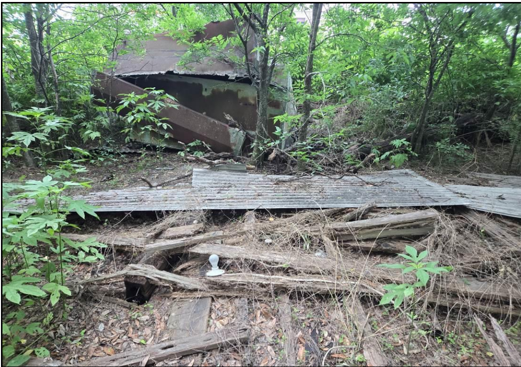
Figure 9: View of collapsed shed/barn facing southwest
