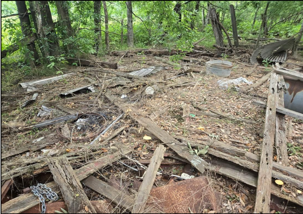
Figure 8: View of collapsed shed/barn facing northeast
